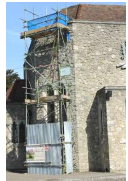
Scaffolding has been erected around the chapels to enable the work on the roofs.
